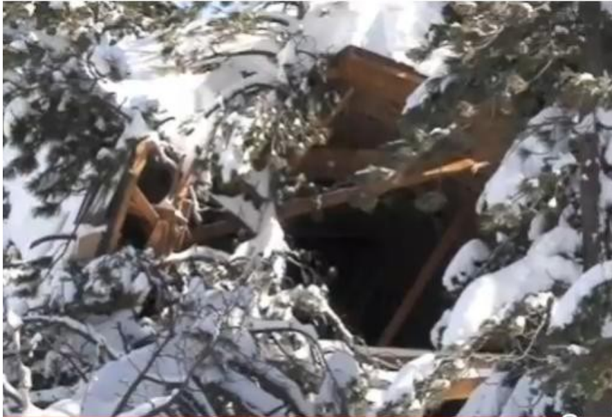
Cabin in Meadow View Heights damaged by the storm before Christmas
